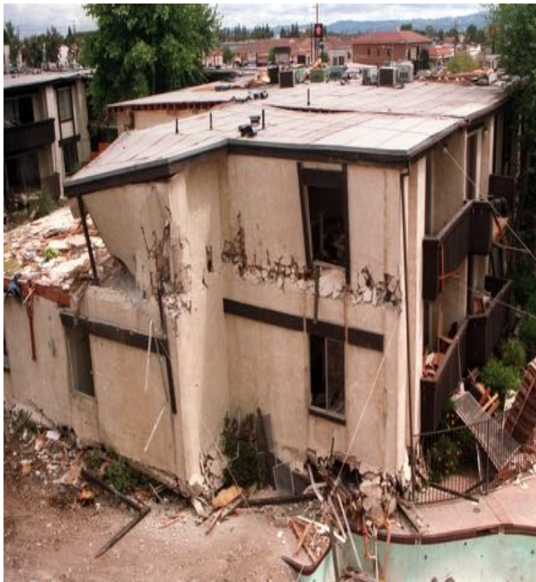
Figure 2-5. The Northridge Meadows Apartments after the January 17, 1994 Northridge earthquake. Source: Los Angeles Times
