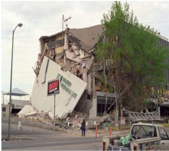
Figure 2-7. The Kaiser Permanente Office Building, a non-ductile concrete building that suffered partial collapse in the January 17, 1994 Northridge earthquake.
