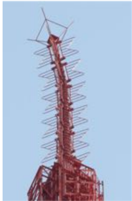
Figure 4-3. Telecommunications tower in Tokyo, damaged in the 2011 Tohoku magnitude 9 earthquake.
