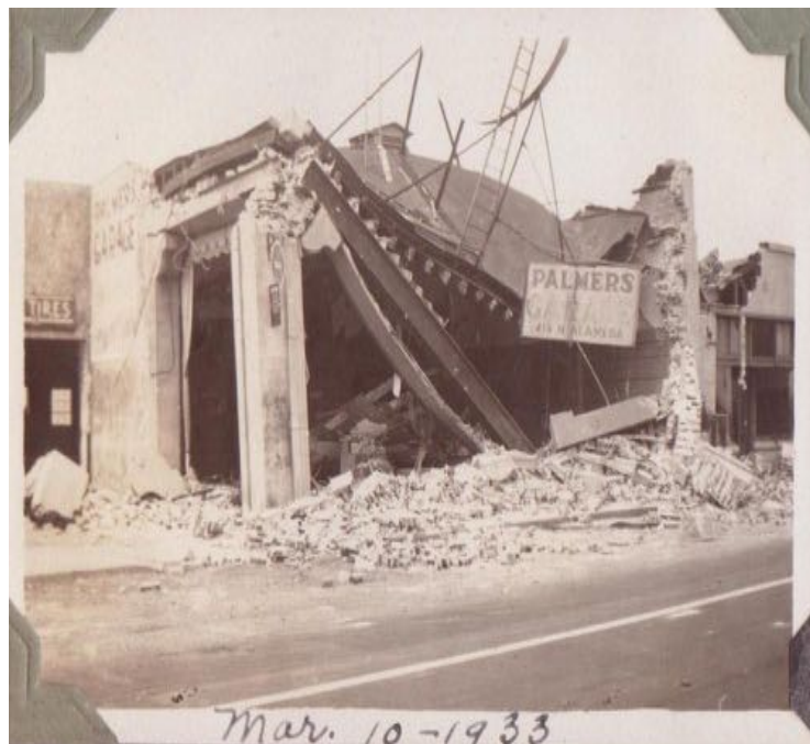
Figure 2-3. Damage to an unreinforced masonry building in the 1933 Long Beach earthquake. Source: USGS
