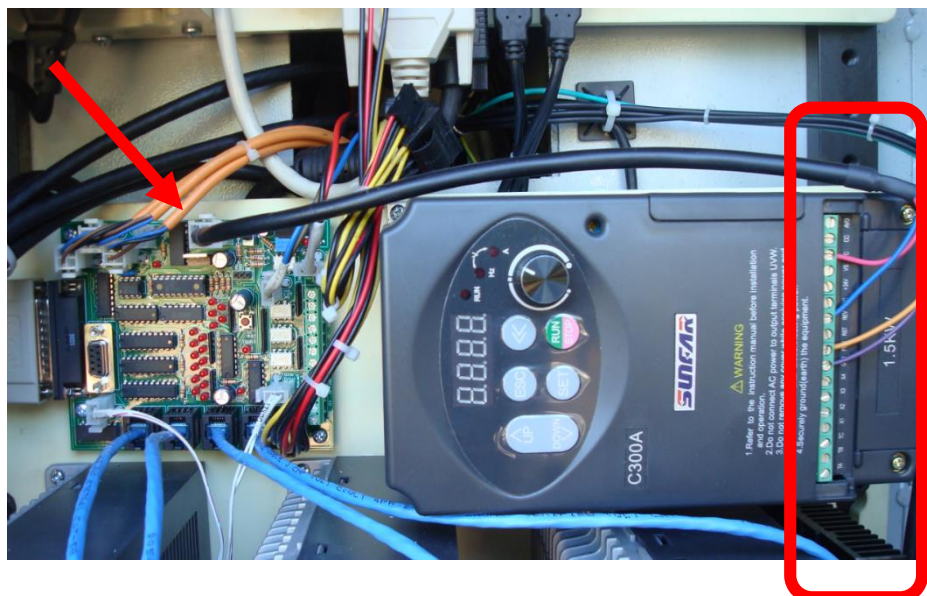
Figure 3-9 BOB and VFD
