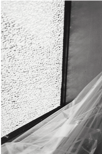
Fig 4 Failure of vertical toughened glass
