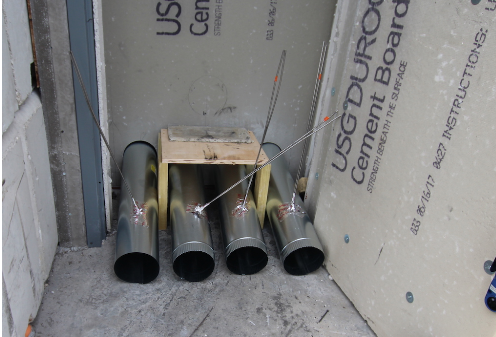
Figure 4.1: Leakage pipes (0.15 m (6 in.) diameter) installed in the side A wall of the basement.
