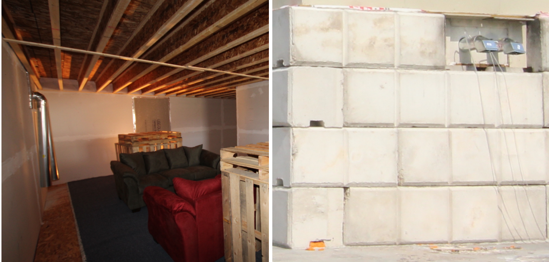
Figure 4.4: Photographs of installed dryer vent from the inside of the basement (left) and outside the structure (right).
