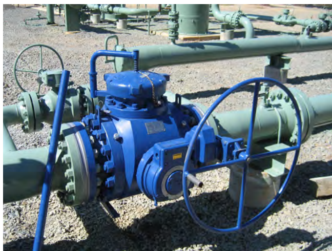
Figure 1. A 10 in. Argus pig valve receiver station in Haynesville Shale Gas, Louisiana (USA).
