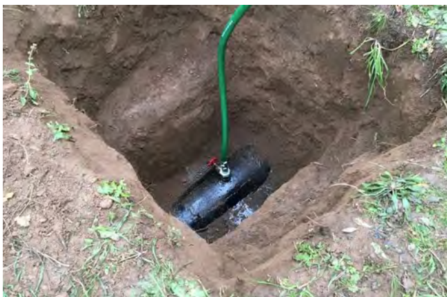
Figure 3. Illegal hot tap detected and localised by the e-vpms waveleak®.
