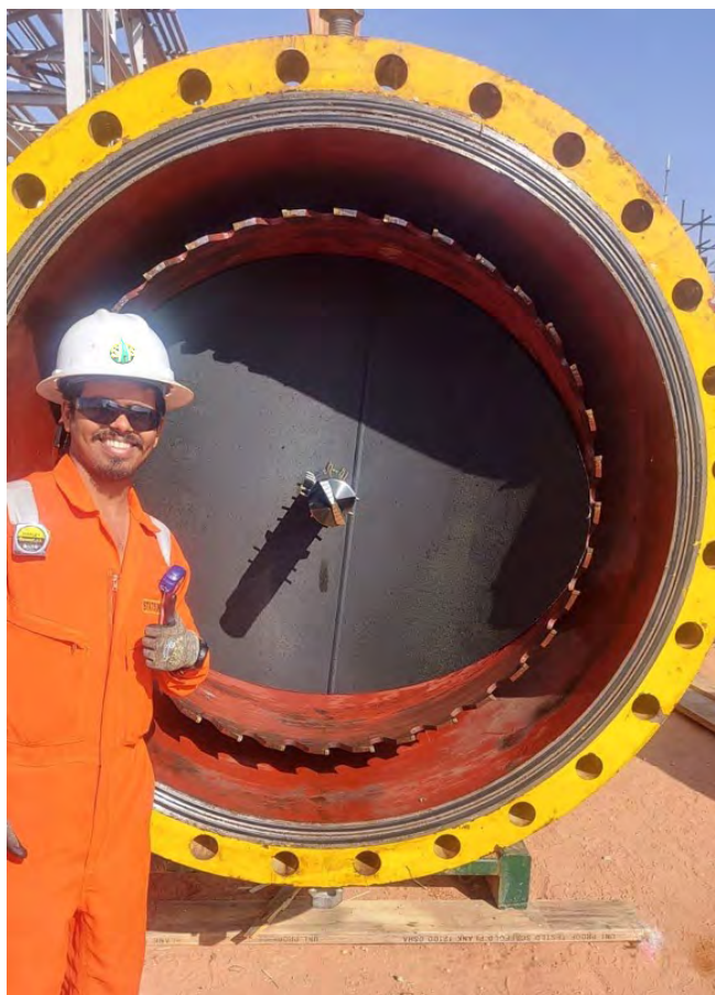
Figure 5. 48 in. SureTap hot tap of crude oil line for BISEP deployment (Saudi Arabia).
