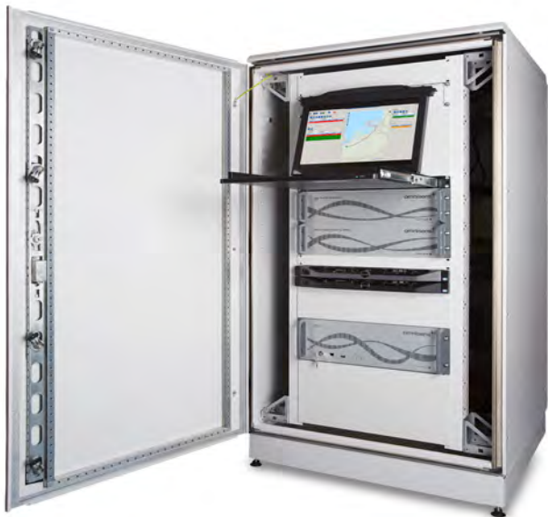
Figure 3. Omnisens LYNX system telecommunication rack cabinet.
