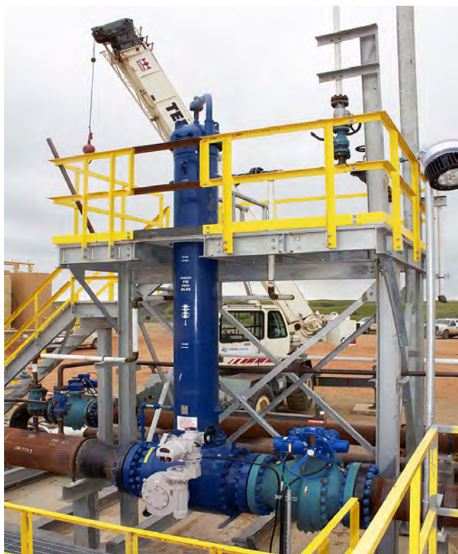
Figure 3. Example of an Argus Multi-Pig Launcher station in the field.
