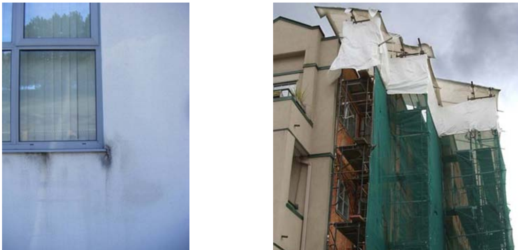
Figure 1.12– Failure due to poor interface detail (left), repairs in British Columbia (right)
