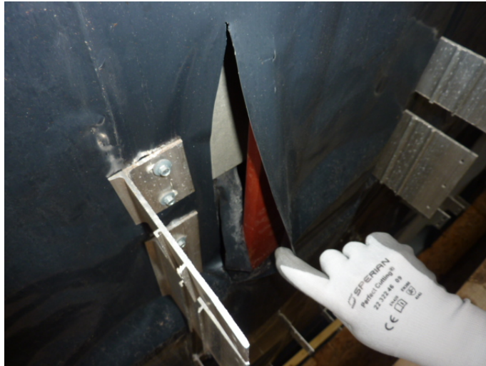
Figure 4.12- Poorly installed/damaged vapour control layer
