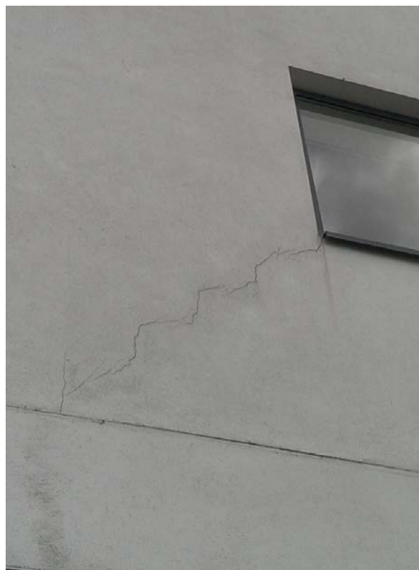
Figure 4.38 – Render cracking at window corner
