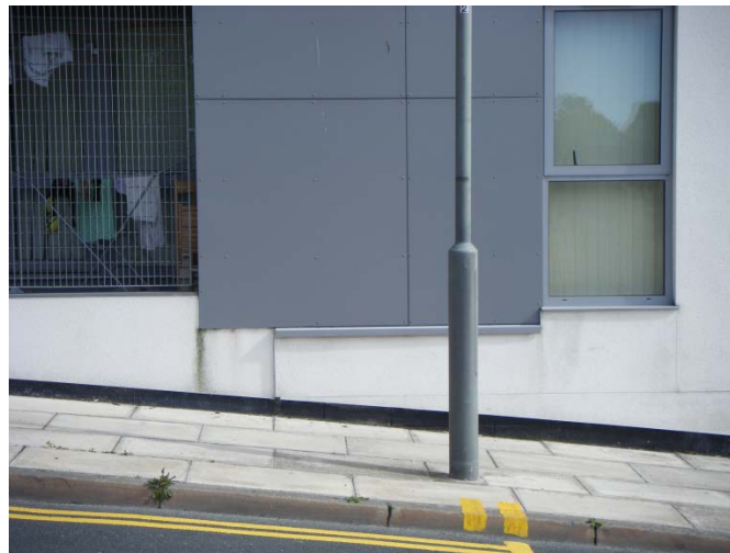
Figure 7.5 - Missing sill/flushing (left)
