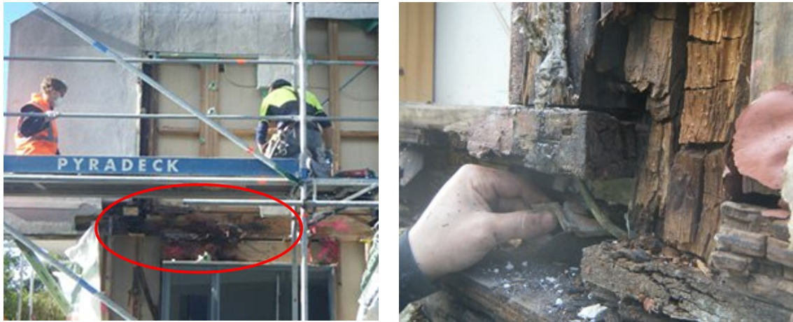
Figure 3.12 – Failure of an external insulation system on a timber frame with no cavity, New Zealand (less than 10 years old)
