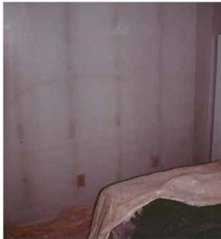
Figure 1.1 - Dust staining on the internal surface at stud locations due to thermal bridging
