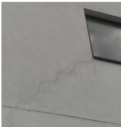
Figure 6.5.6 – Cracking in render at a re-entrant corner
