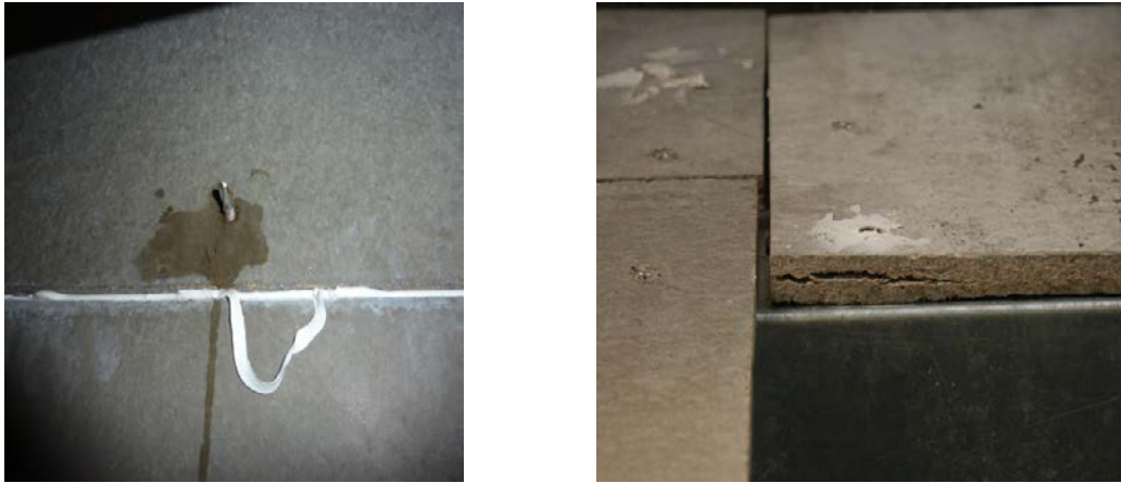
Figure 4.5 - Fixing into sheathing causing water penetration, poor workmanship when sealing the boards (left), damage during fixing (right)
