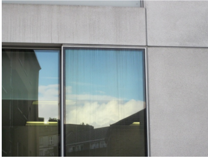
Figure 7.4 - Run-off from concrete causing staining on glass below
