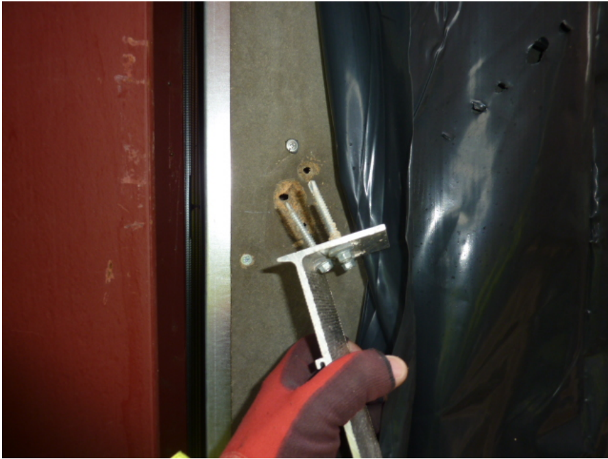
Figure 4.29 - Fixings into the sheathing board rather than the steel stud
