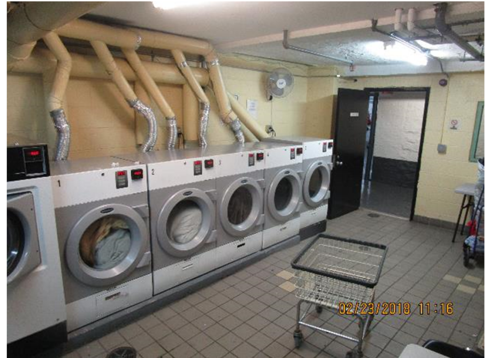
1000s of CFM of exhaust in this room
