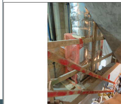
Notes: Duct insulation (indoors)
