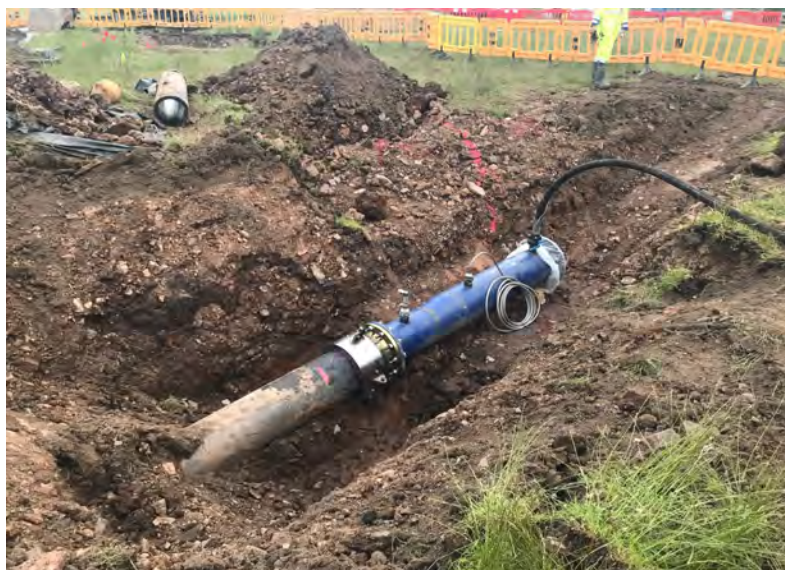
Figure 5. 14 in. x 12 in. temporary pig launcher onsite.
