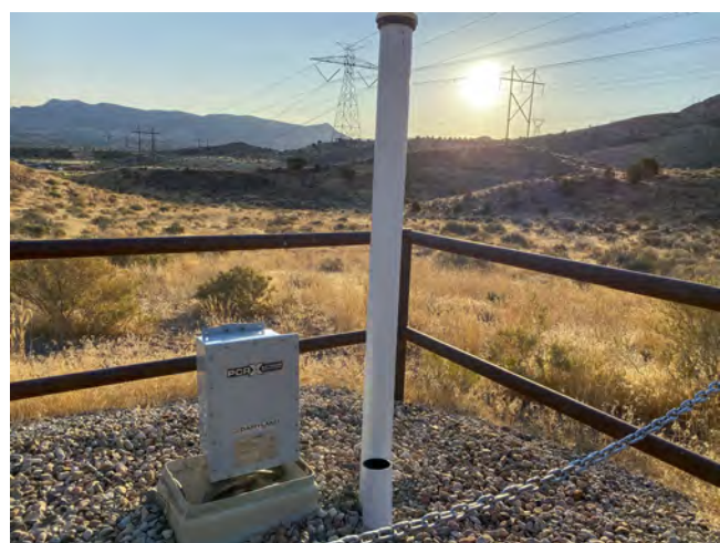
Figure 6. A Dairyland PCRX decoupler installed as part of an AC mitigation system.
