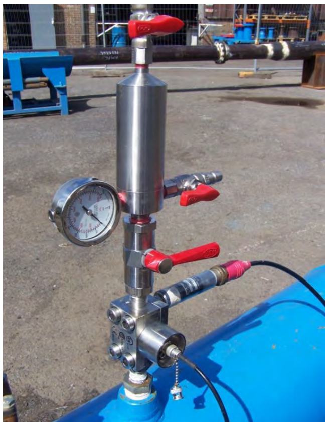
Figure 1. Acoustek blockage detection system connected to the pipeline.
