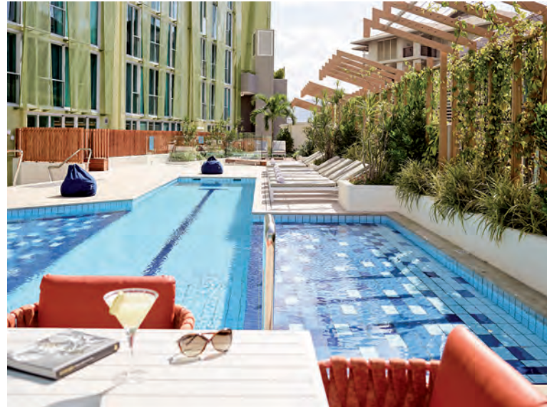
The substrates of the pools of the complex were waterproofed with MAPELASTIC SMART, before installing ceramic tiles with KERAFLEX MAXI S1 and grouting the joints with KERAPOXY.
