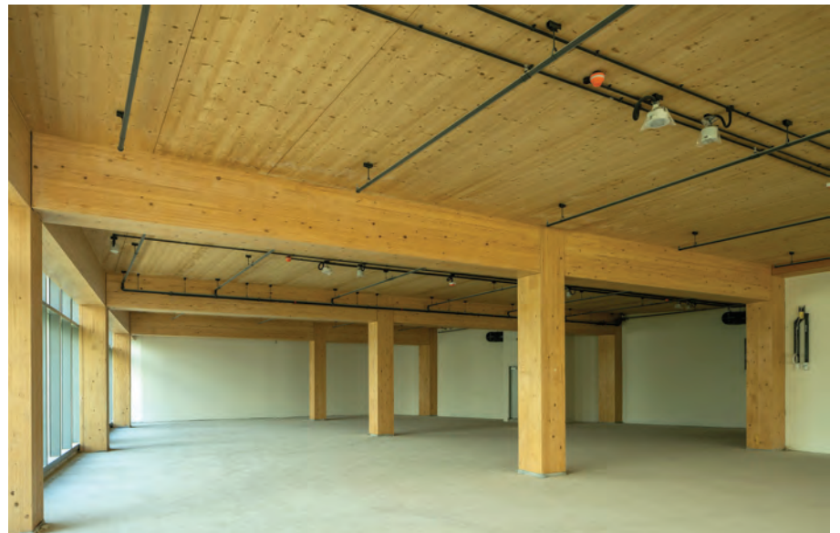
Apart from being environmentally sustainable, the MET was fabricated off-site, providing better construction quality control and higher productivity with 60% reduction in on-site manpower, compared to traditional construction methods.
