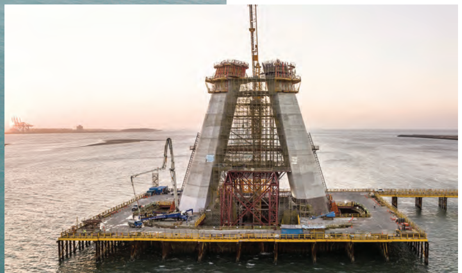
ABOVE AND LEFT: The pylon in the centre of the bridge is a highlight. It towers into the air in the shape of an upturned 'Y' and stands, figuratively speaking, with its two legs in the river. The stay cables, which run in parallel to the top of the pylon from both sides, give the structure a futuristic appearance.
