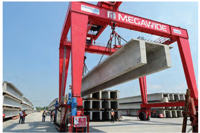
Philippine contractor Megawide's PCS unit is supplying precast double-tee slabs for the North Luzon Expressway's (NLEX) Candaba Viaduct expansion project.
