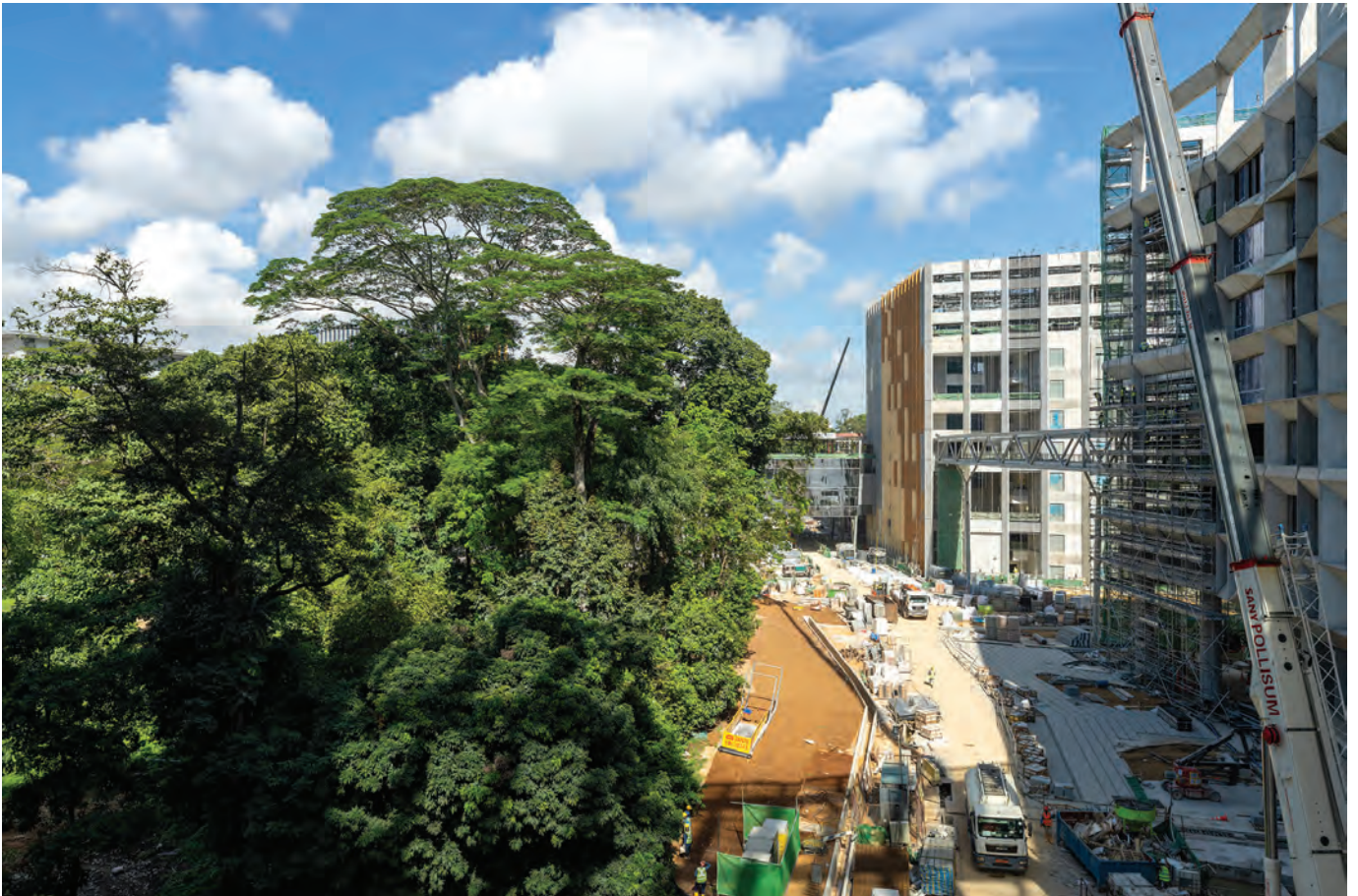
Heritage Trail under construction. To build a highly liveable environment with regenerative landscapes, Punggol Digital District actively conserves the site's natural assets by pedestrianising the existing old Punggol Road into a 1.3 km tree-lined Heritage Trail.
