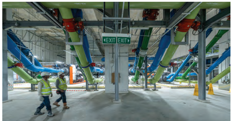
The district cooling system provides chilled water centrally to multiple users across all buildings in the district, including business park, office, retail, hotel/serviced residence, SIT Punggol Campus, transport facilities and community amenities.
