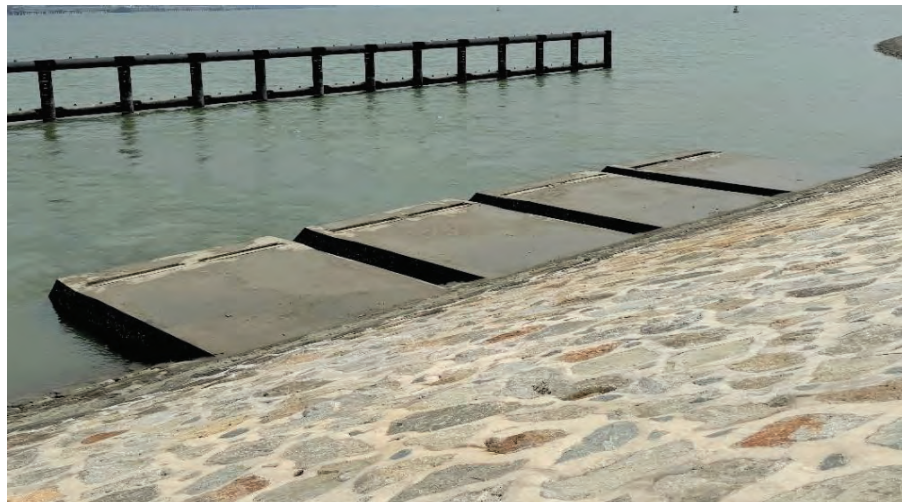
BELOW: Multiple outlet structures run through the coastal dike and help channel excess water from the polder out into the sea.
