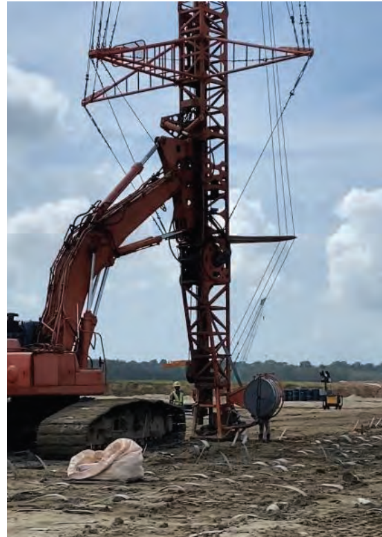
Prefabricated vertical drains (PVDs) were inserted to drain water out of the clayey soil. The process transformed the soft soil into sturdy usable land, ready for development.
