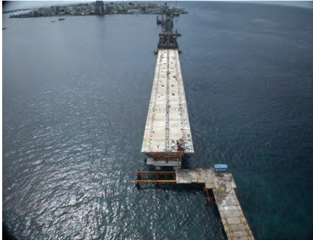
ABOVE: Currently under construction, the Greater Male Connectivity Project (GMCP) will link Malé, Villingili, Gulhifalhu and Thilafushi through a 6.74-km network comprising three navigation bridges, deep and shallow water marine viaducts, and at-grade roads.
