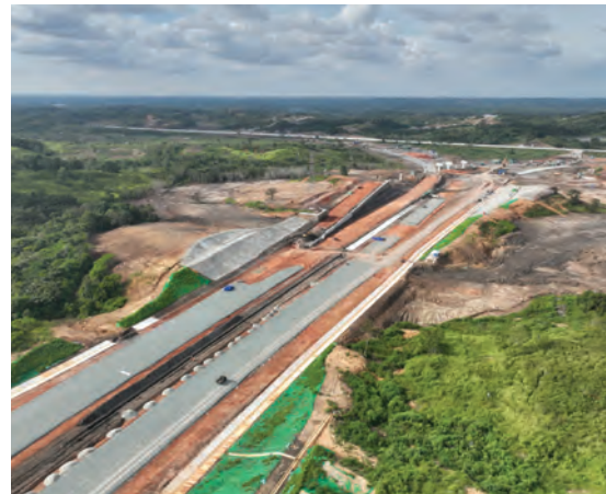
The IKN Section 1B Toll Road project uses various technologies, and also focuses on sustainability and social benefits.
