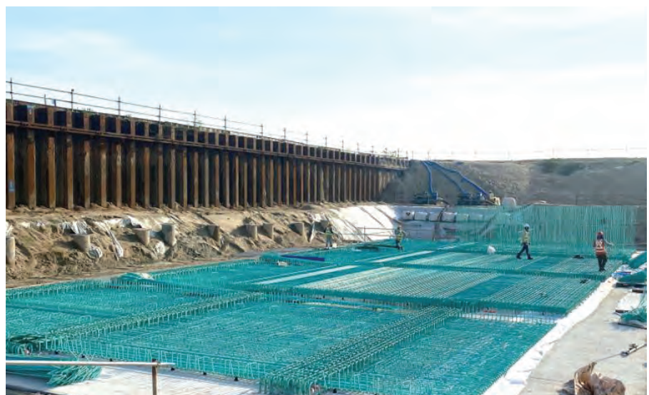
Cofferdams were installed to keep the construction areas of the outlet structures sufficiently dry, before the coastal dike was built over the completed outlet structures.
